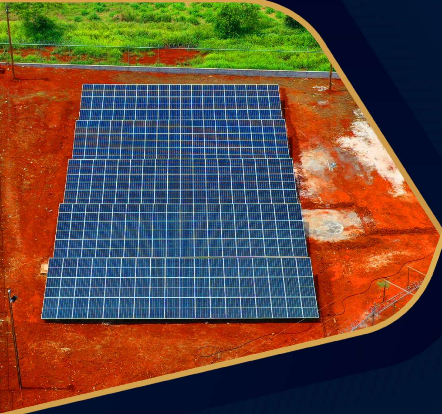
BEACON E SORAL PLANT
