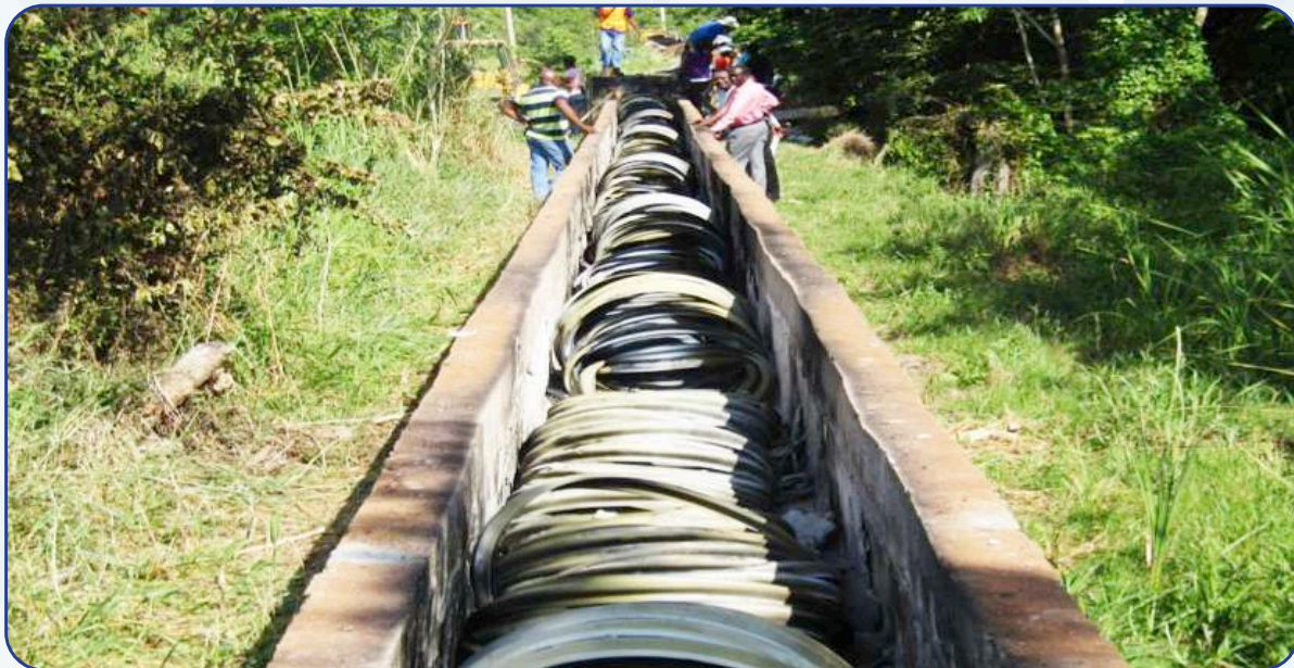
Arson - Destruction of 104 meters of HDPE in the parish of Clarendon
