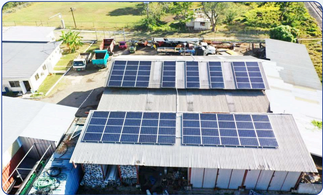
20kW Solar Retrofit of the St. Dorothy District Office in St. Catherine
