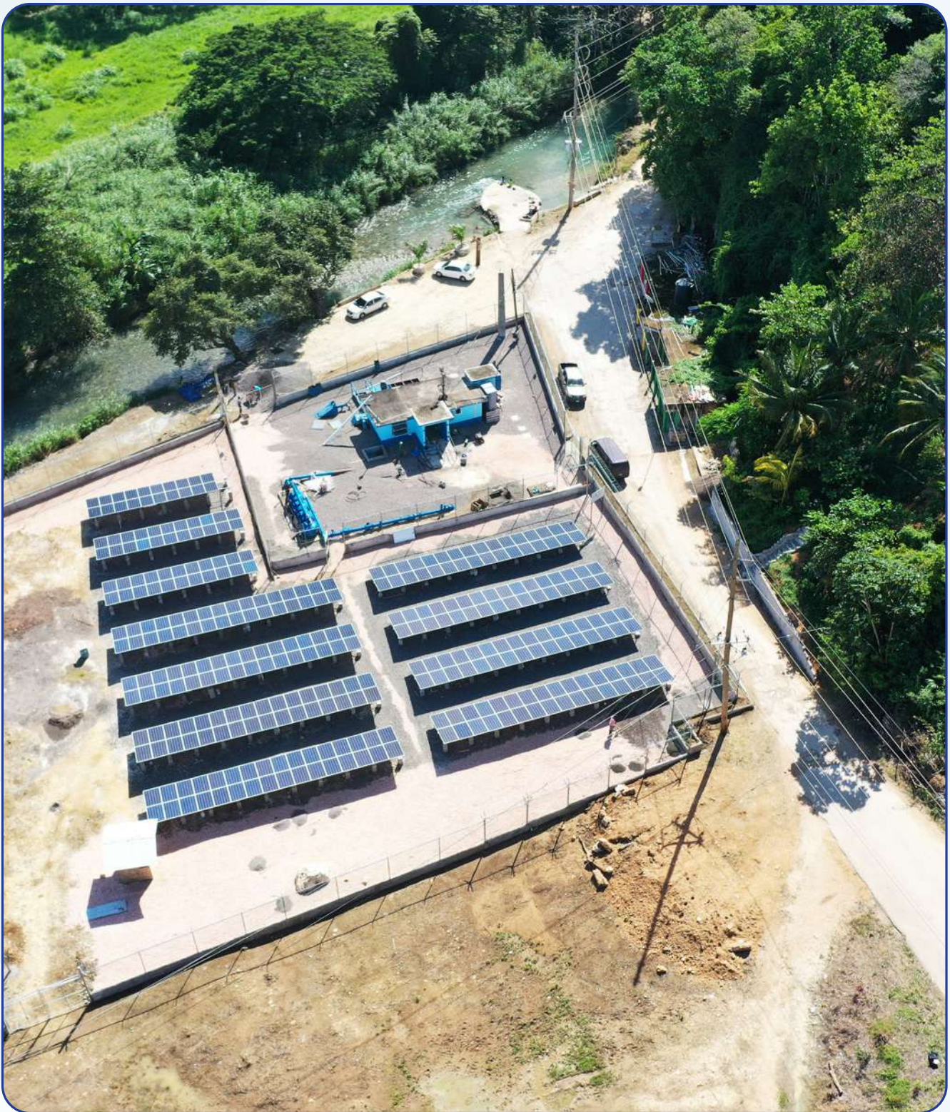
90kW Solar Retrofit of the Bengal Pump Station in Trelawny
