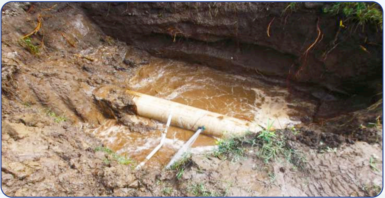
Illegal abstraction of water from the NIC pipeline 5 feet underground, in the parish of St. Thomas
